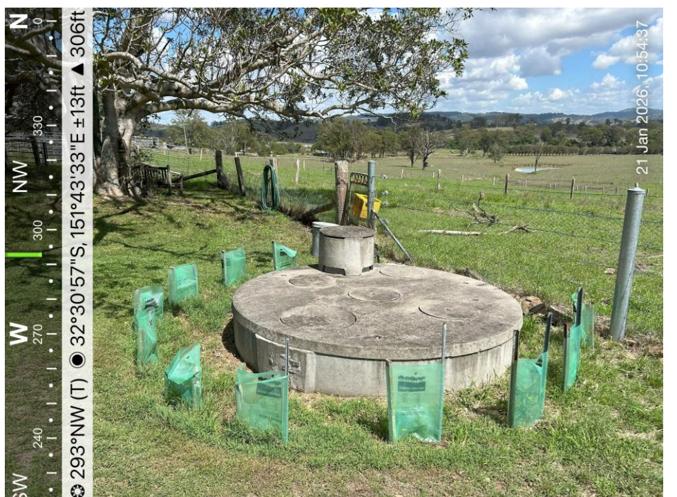
Photo 10: Overview of the underground septic tank adjacent to the northeastern side of the residential dwelling.
